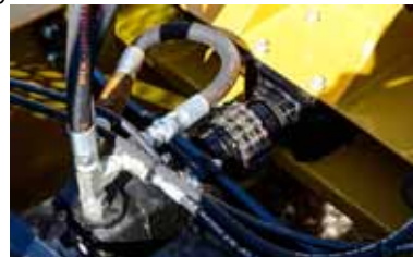
Auxiliary electrical connection
